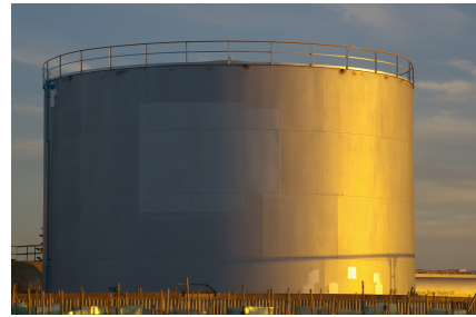
Figure 1: A typical AST this paper is concerned with (aprox. 12,600 oil barrels, found in North Fermantle, AU)
